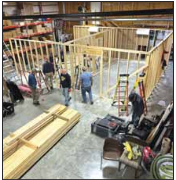
When the BDM Dawson Springs site closed, the temporary “cube” that was built specifically for housing BDM volunteers was torn down. This makes room for Habitat to return to regular operations in the building. courtesy of BDM
